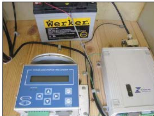
Flume equipment box with flume flow discharge read-out. Radio or satellite signals are relayed by antennas from the flume data recorders and received by remote computer in Santa Fe every 15 minutes. Office of the State Engineer/Interstate Stream Commission uses the flow data to assist in administering water rights and managing water throughout the state.
