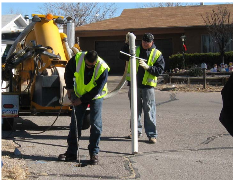
Figure 10: Personnel cleaning out valves prior to logger deployment
