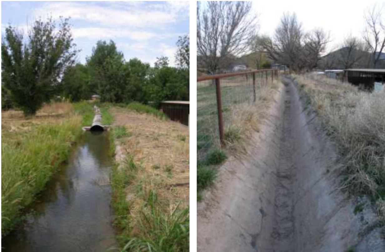
Figure 5. Before and after photos of a degraded section of Pleasanton East-side Ditch that PEDCo recently repaired by inserting closed pipe. For reference, note the same tree appears upper left in both photos.
