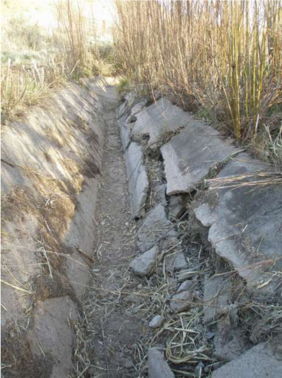
Figure 3. Typical reach of East-side Pleasanton Ditch showing 50 year-old degraded concrete lining which contributes to conveyance loss through leakage and seepage.
