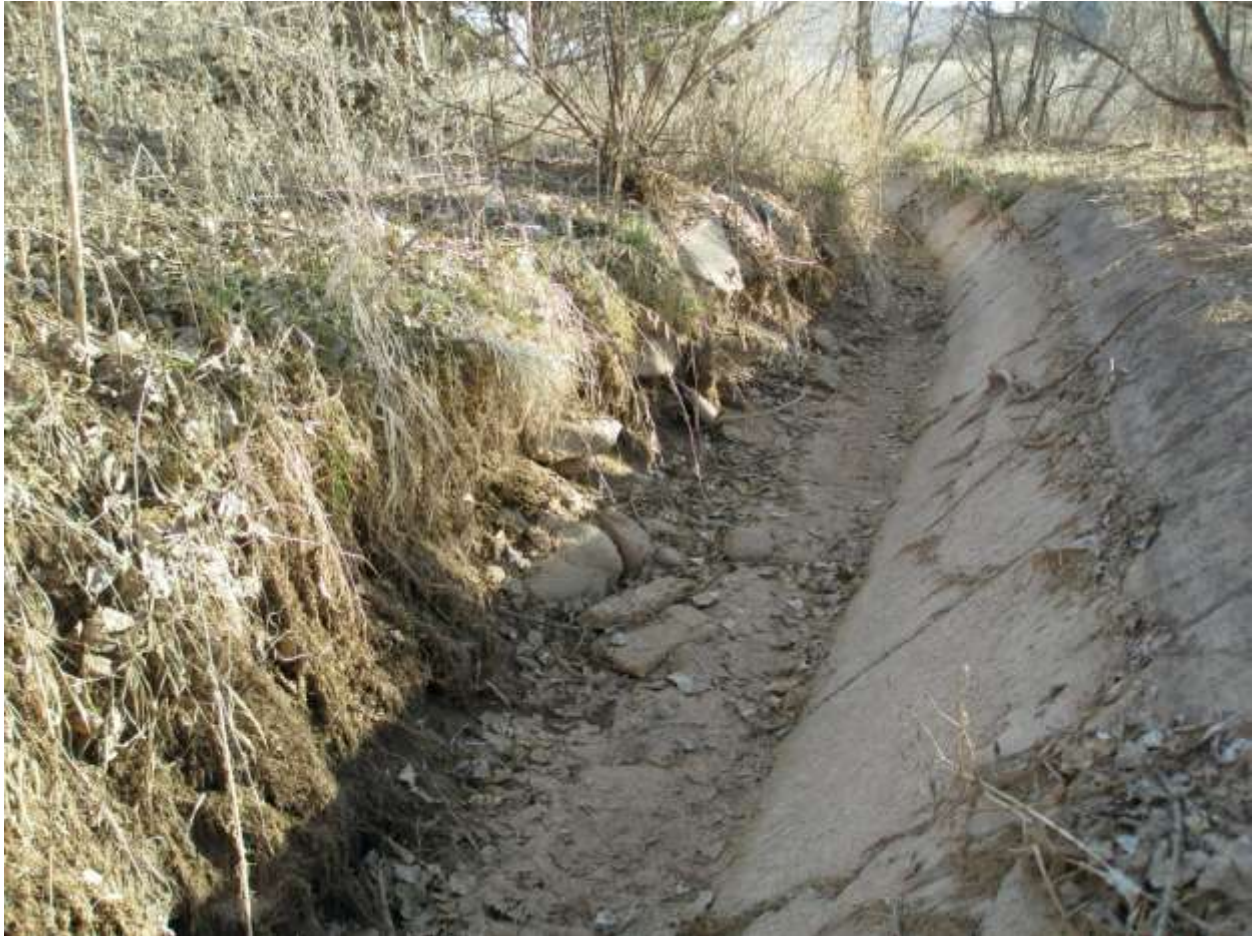
Figure 4. Bank lining of this section of East-side Pleasanton Ditch is completely degraded and contributes to conveyance loss through leakage and seepage.
