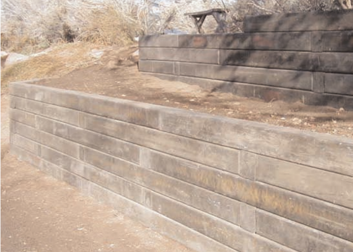
Figure 1-3: Retaining walls are an effective way to create terraces to control erosion and create spaces for plants.
