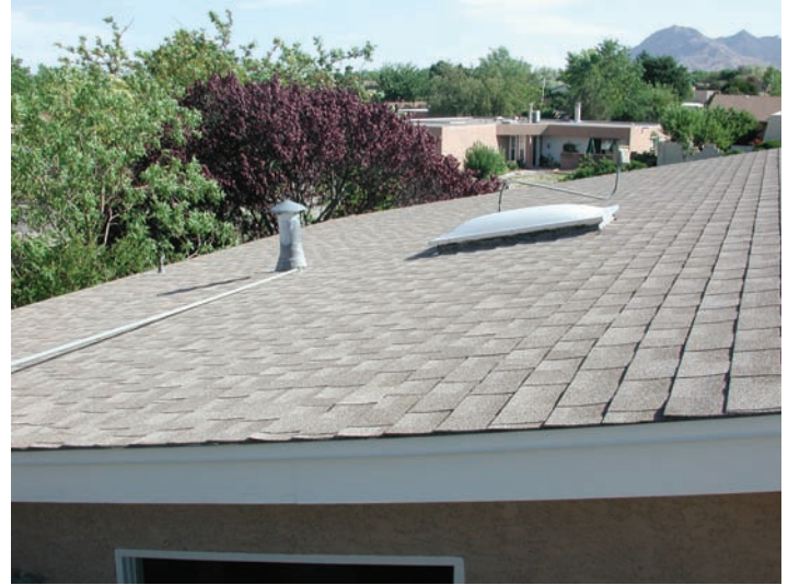
Figure 7-3: Asphalt shingle roofs, which are popular because they are relatively inexpensive, can be efficient for water harvesting.
