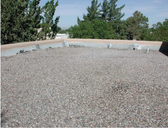
Figure 7-2: Although not the most efficient surfaces for harvesting rainwater, flat roofs can serve well as catchment areas for roof-reliant landscaping systems.
