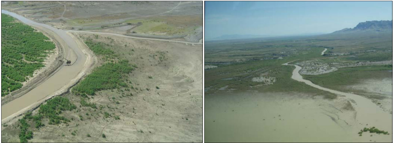
Excavation of the Elephant Butte pilot channel reconnected the Rio Grande with the lowered reservoir pool following several consecutive years of drought.
