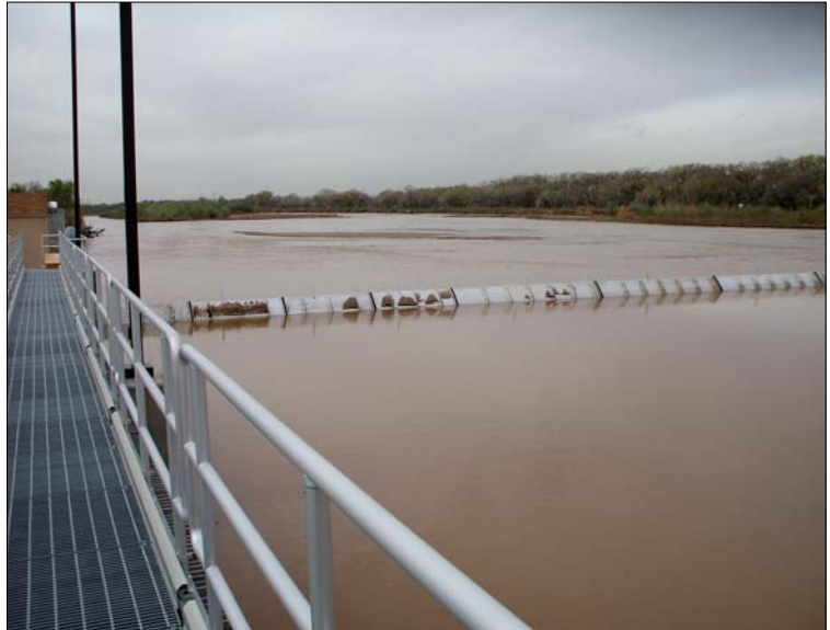
Albuquerque's newly constructed diversion dam will allow the city to tap its San Juan-Chama water for municipal drinking water supply use.
